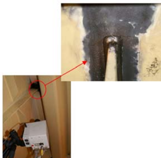
Fig. 7 Crack detection in actual steel bridge.
